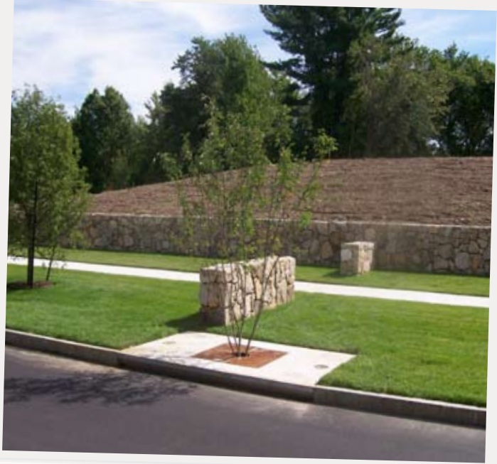
Several Filterra units were installed along Southfield's, Shea Blvd. to meet stormwater quality regulations and Smart growth practices.
