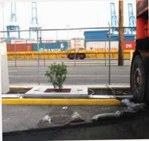
Filtterra's small footprint made for simple installation at the Port of Tacoma.
