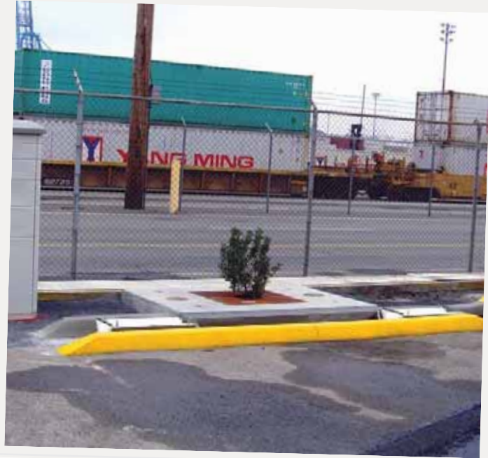
A Filterra Bioretention System was installed at Port of Tacoma to help mitigate the amount of TSS, heavy metals, nutrients and bacteria from entering the Puget Sound.
