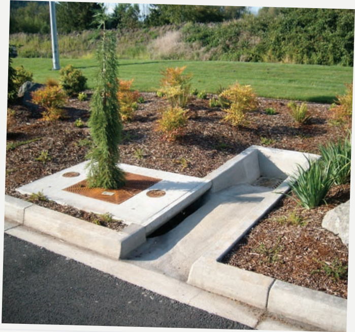
Two Filterra Bioretention Systems were installed in the parking lot of the Jamestown S'Klallam Tribe's Longhouse Market to meet state goals for waterway protection.
